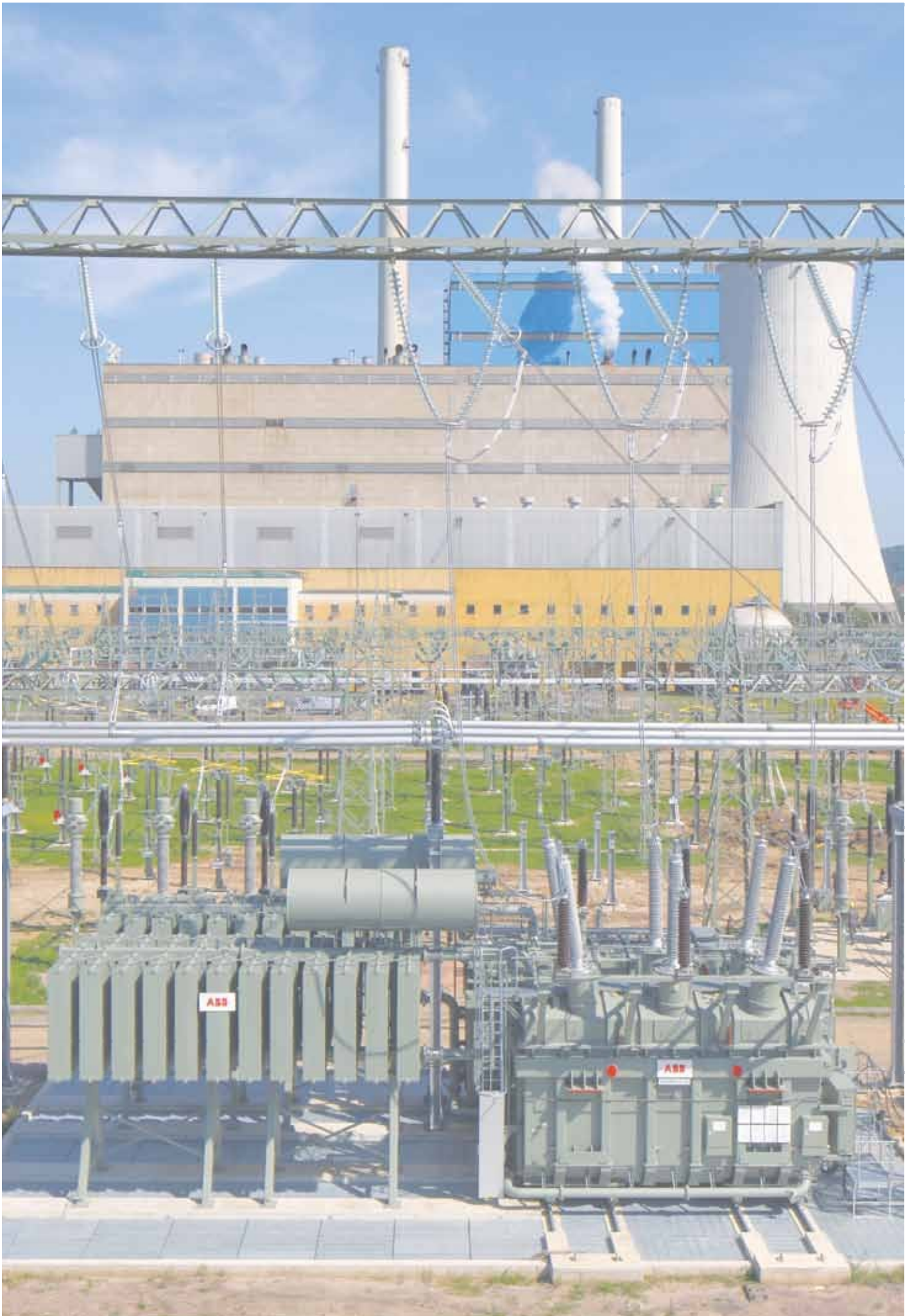
2 Phase shifting transformers
